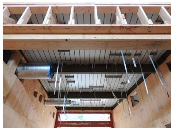
Mechanical unit and ductwork installation in progress at the upper level "Eddy".
