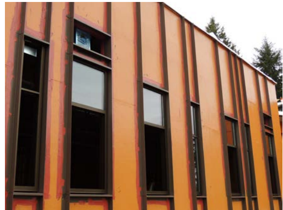
Fiber cement board siding trim and glazing installation in progress, East Elevation.
