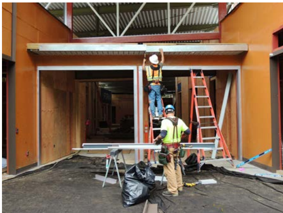
Sheet metal flashing installation in progress at the "Outdoor Deck" entry, upper level.
