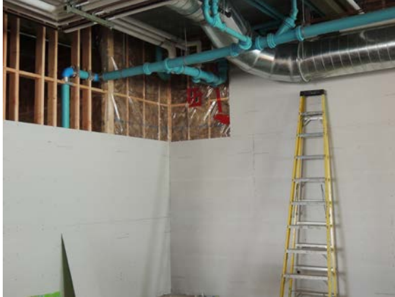
Gypsum wallboard installation in progress at the "PDZA Staff" room, lower level
