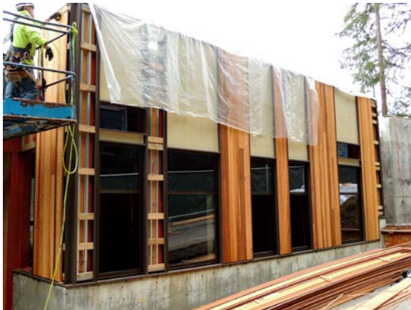
Glazing, wood cladding and fiber cement board siding installation in progress, West Elevation.
